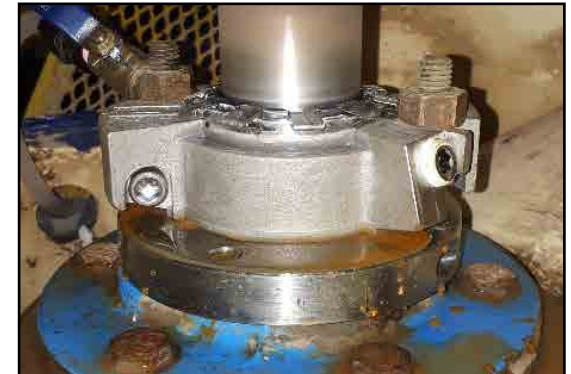
The split seal is running effectively with no maintenance required.
