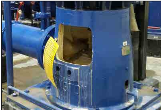
The pump shafts were extremely damaged.
